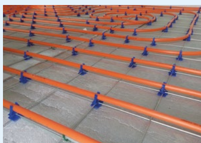
Exemple of heating system
